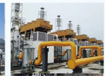
◆ Distributed energy generation
